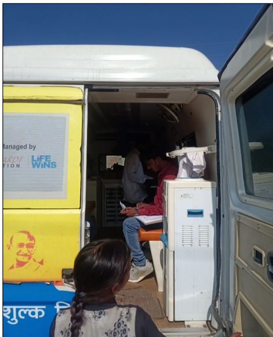
Figure 19: RO water system in MMU van
